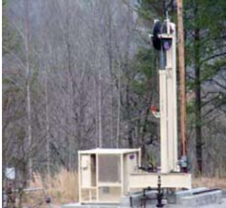
DynaPump Model 7 operating in Alabama
