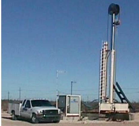
DynaPump Model 9 operating in West Texas
